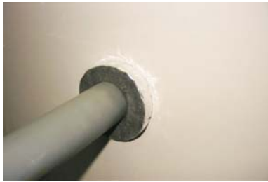
Fire sleeve fitted into wall
