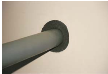
Clean wall solution
